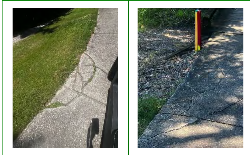
2024 images showing cart paths in need of repair.
